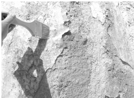
Figure. 1 Plaster whit loss of cohesion
