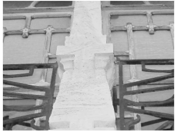
Figure 9. Column granular disintegration
