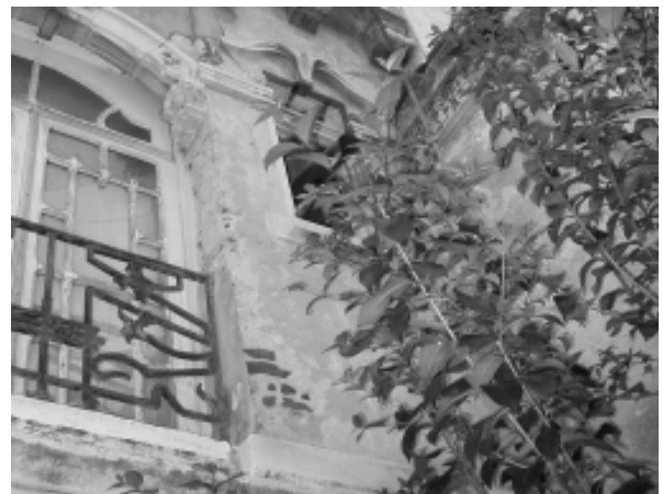
Figure 10. Areas of missing render
